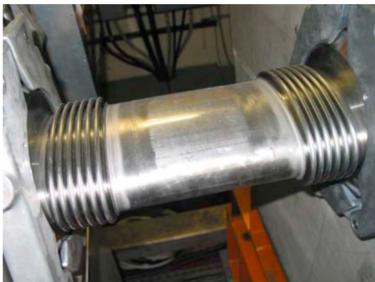
Ovale Kompensatoren im Beschleuniger des CERN Oval expansion joints installed at the accelerator at CERN
