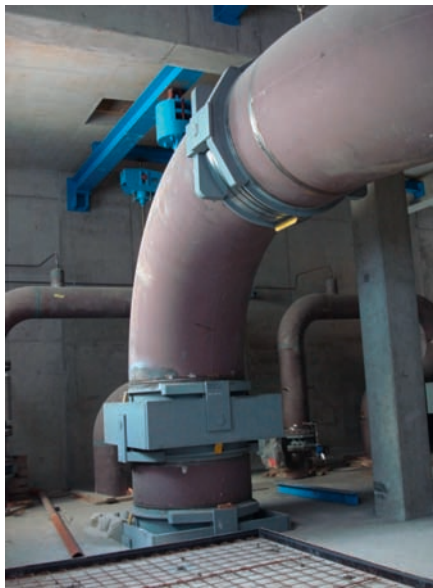
Kardan Kompensatoren in einem Kraftwerk Kardan expansion joints installed at a power station
